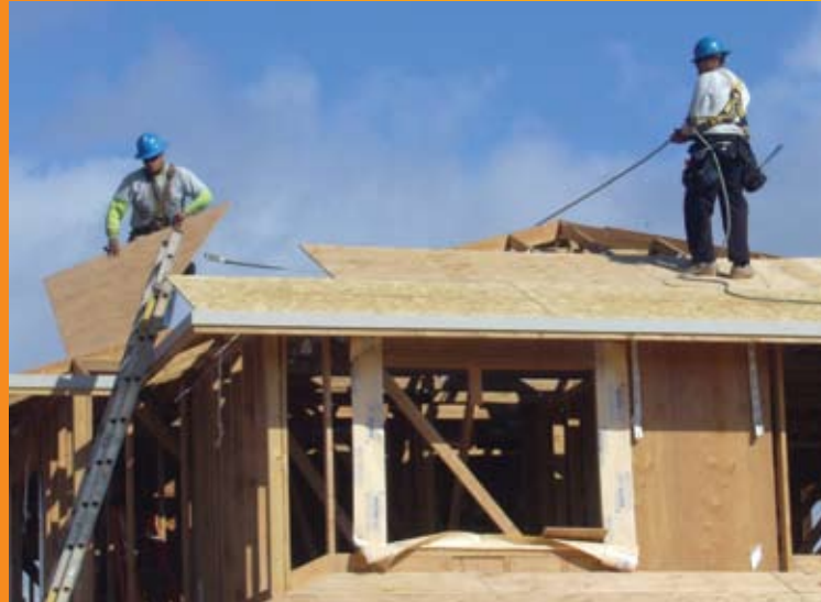
A Gentry Homes crew observes safety measures at DHHL's (Department of Hawaiian Home Lands) Kanahili Phase 2 project in Kapolei. Gentry is a client of Risk Solutions Partners.
