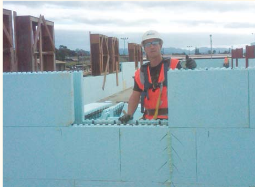
Andy Hahto of Absher Construction Company, a Lawson & Associates client, installs an ICF (insulating concrete forms) wall at a Schofield Barracks complex project.
