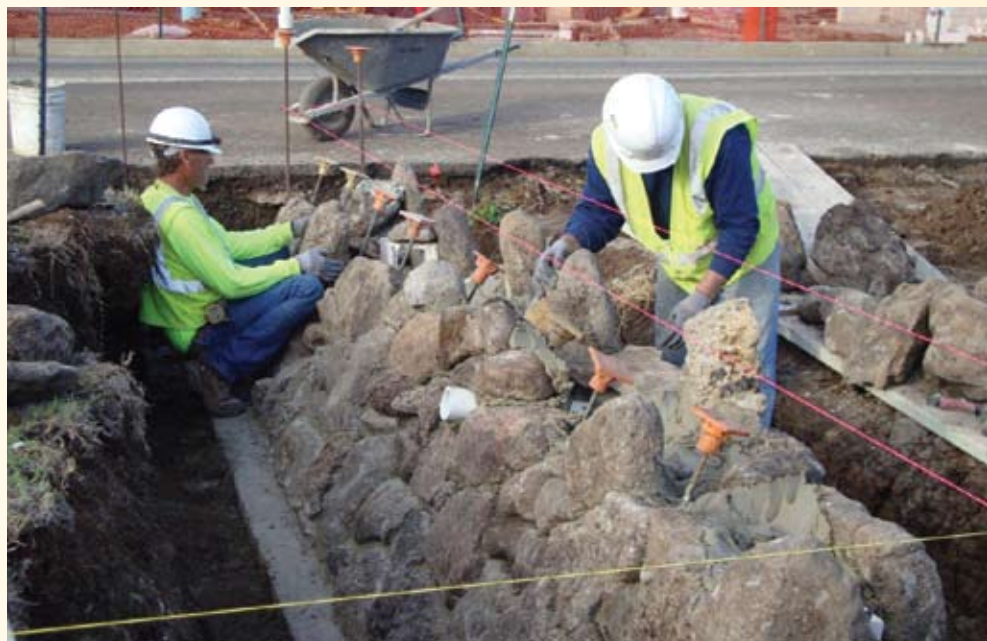
Lyle Hoffman and Kevan Sutch of San Juan Construction, another Lawson & Associates client, work on an Army Reserve project at Fort Shafter.
